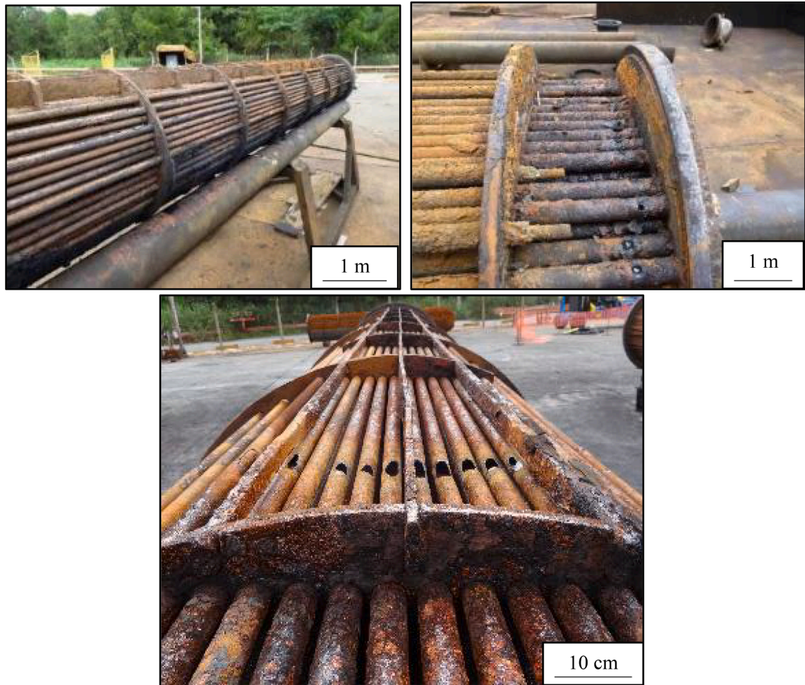
Fig. 6. External visual analysis of the load heat exchanger tube bundle (E-0004).
